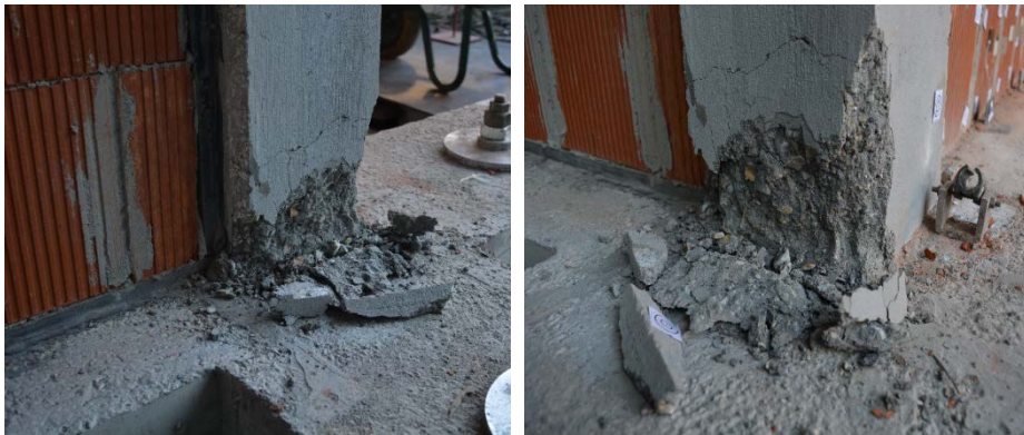
Figure 61: Spalled concrete cover of the column in the bottom
