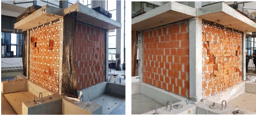
Figure 60: Final state of damage – Phase A
